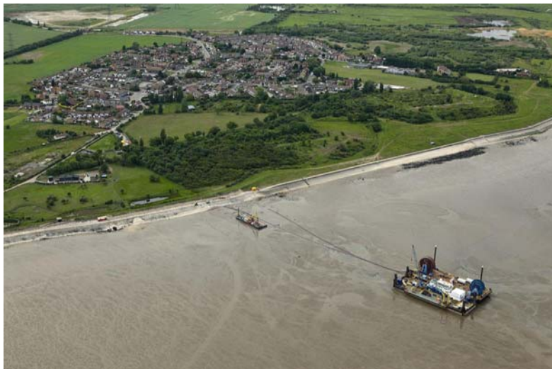
Figure 4-D : BritNed inshore installation spread – the Fetsy L multi-role and Stemat 81 flat barge
